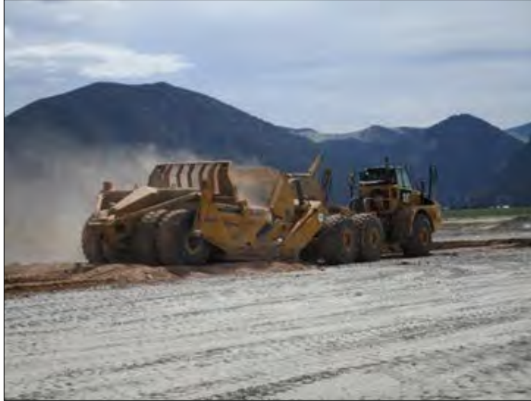
Preliminary work on tailings pond reclamation at the Questa Mine, Taos County (2019)
