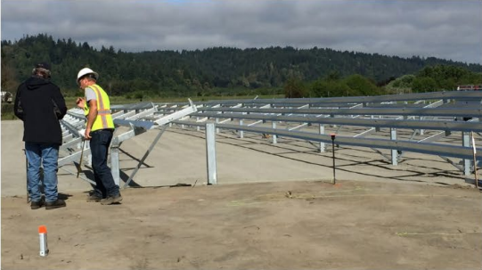
Workers installing the racking for the Blue Lake Rancheria's 500-kilowatt solar system in June 2016. The solar system is a cornerstone of the tribe's low-carbon community microgrid project.
