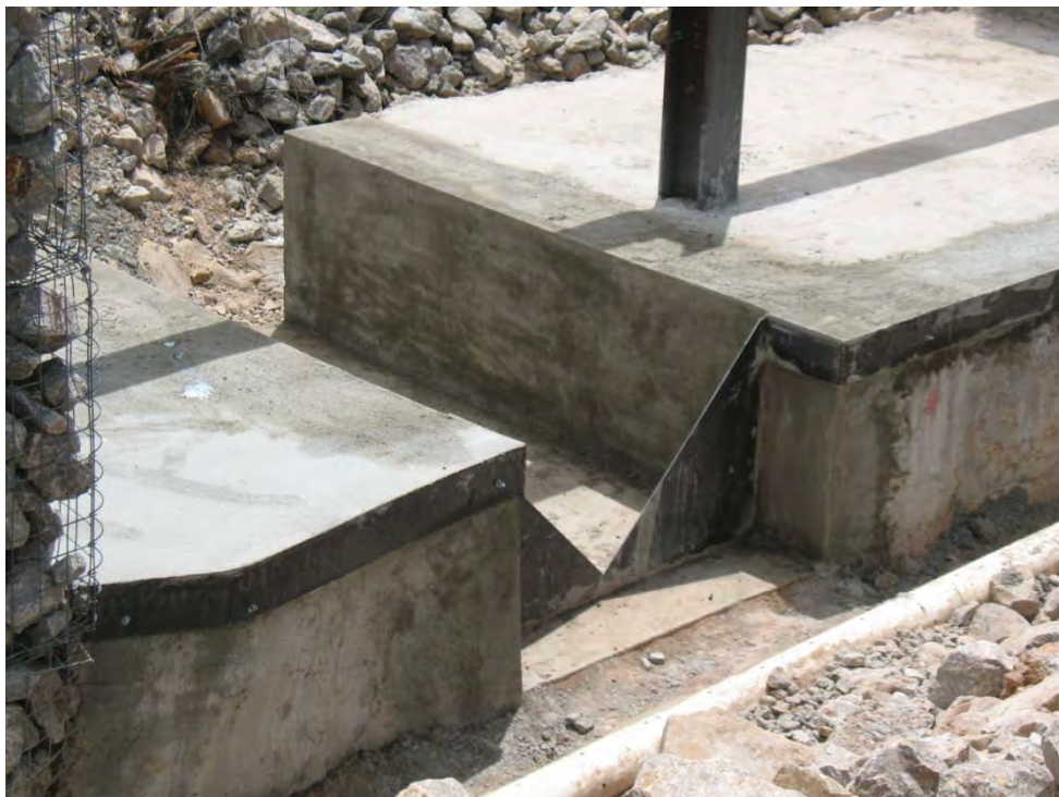
“V” notch weir, new concrete channel and steel “leading edge” of weir construction complete.
