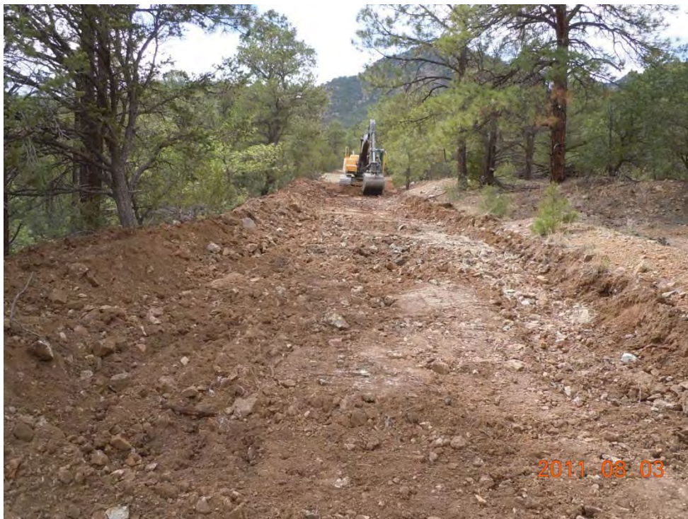
Roadway north of main channel and filled low area reconfigured to prevent flow onto filled area.
