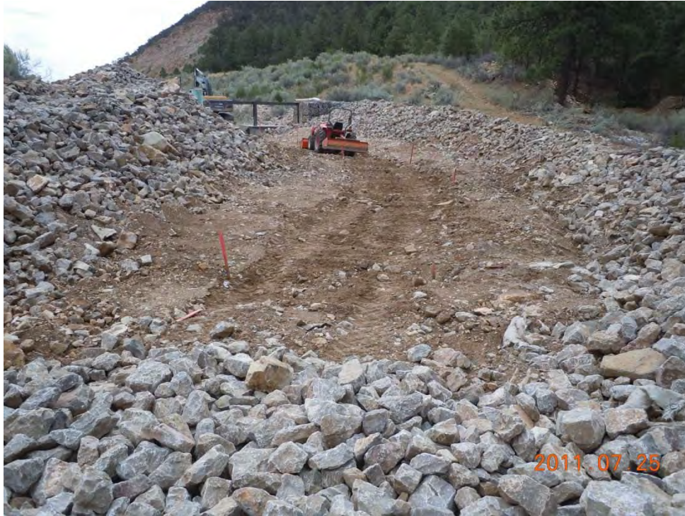
Channel upgradient of weir construction to slope at 1 ½ % and prepare for liner.
