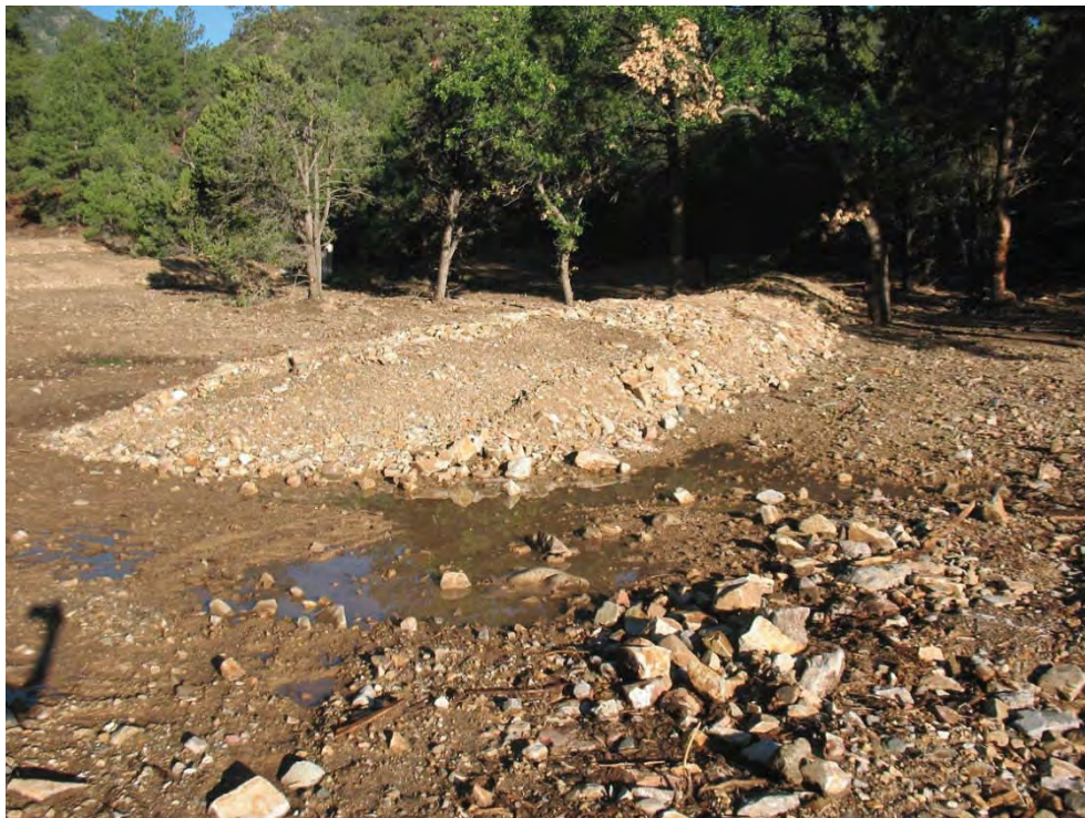
Upgradient area with oversized “waterbars” at completion of construction and after 2 inch rainstorm.
