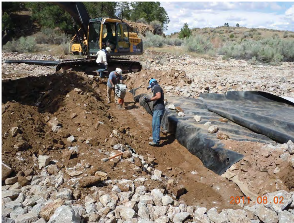
“Leading edge” 3 foot deep anchor trench for liner being compacted in 12 inch lifts.
