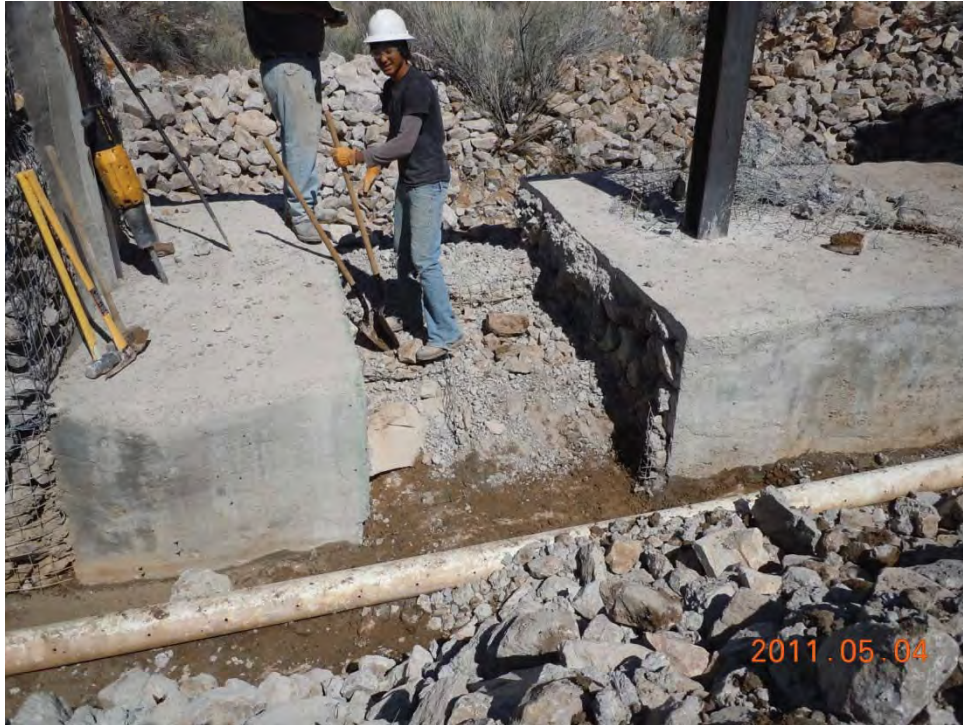
Channel demolition in existing concrete, gabion & riprap for construction of new “V” notch weir.
