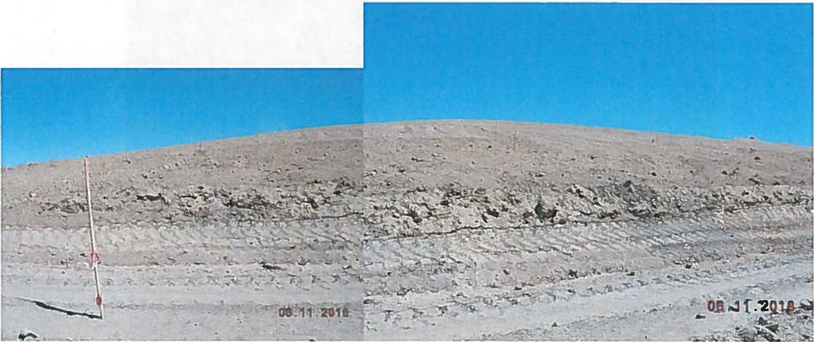
South facing waste rock pile rough graded to approx. 5H:1V gradient (brown color shaft muck)
