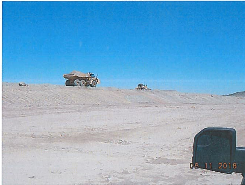
Haul truck delivering excavated waste rock to berm area of Disposal Cell (dozer in background spreading waste rock material for the berm)
