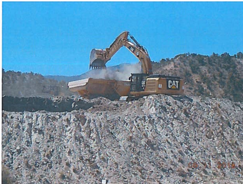
Cat excavator loading waste rock (gray color) from waste rock pile into haul truck
