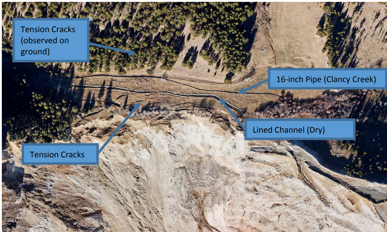
Figure 5. Montana Tunnels Open Pit Highwall Failure Along Clancy Creek. (Photo by Christopher Boyer)
