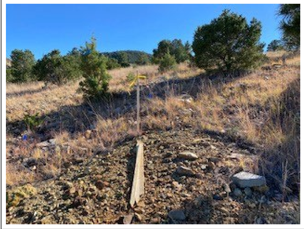
15. WRP location 8 prior to completion of repairs
