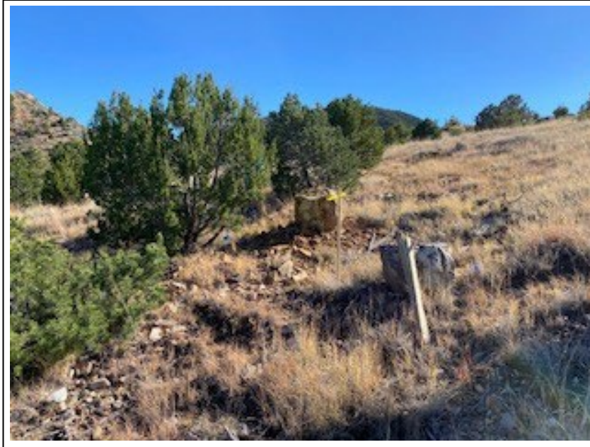
13. WRP location 7 prior to completion of repairs
