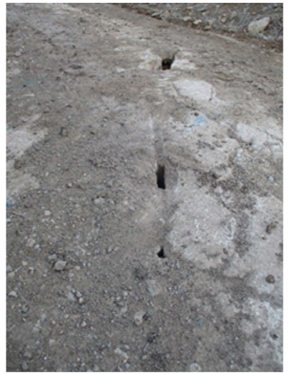
B COUNTY ROAD A-25 SUBSIDENCE FEATURES SCALE: NONE
