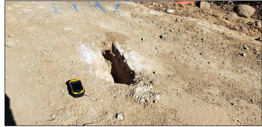
A COUNTY ROAD A-25 SUBSIDENCE FEATURE SCALE: NONE
