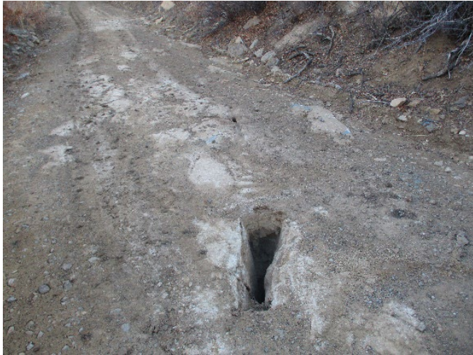
Photo 25. Subsidence features in County Road A-25; February 16, 2022.
