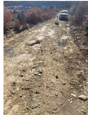
Site photo above the crack looking down the road to the other end of the scan area.
