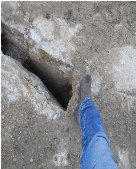
Photo 23. Largest subsidence feature in County Road A-25; February 16, 2022.
