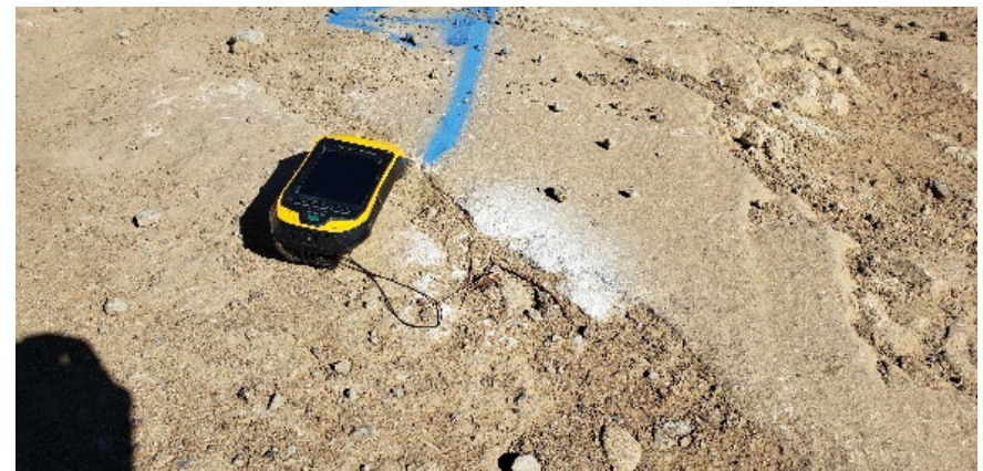
Photo 12. Logging subsidence features in County Road A-25 with GPS unit.
