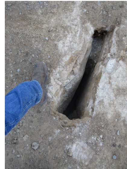
Photo 24. Largest subsidence feature in County Road A-25; February 16, 2022.
