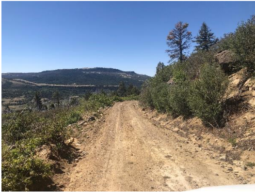
Photo of scan area. Section of road following second bend and containing crack discovered by client.
