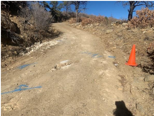
Closer photo of the crack and area of concern, in this photo you can see the blue lines indicating a similar reaction of right over the crack, possibly where the crack is continuing.
