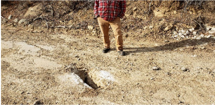
Photo 1. Subsidence feature found by Colfax County Road Department
