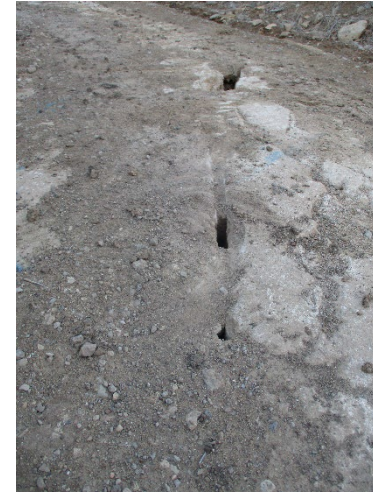
Photo 22. Subsidence features in County Road A-25; February 16, 2022.
