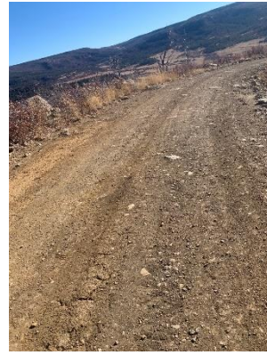
Site photo of the scan area above the rocky area with the crack.
