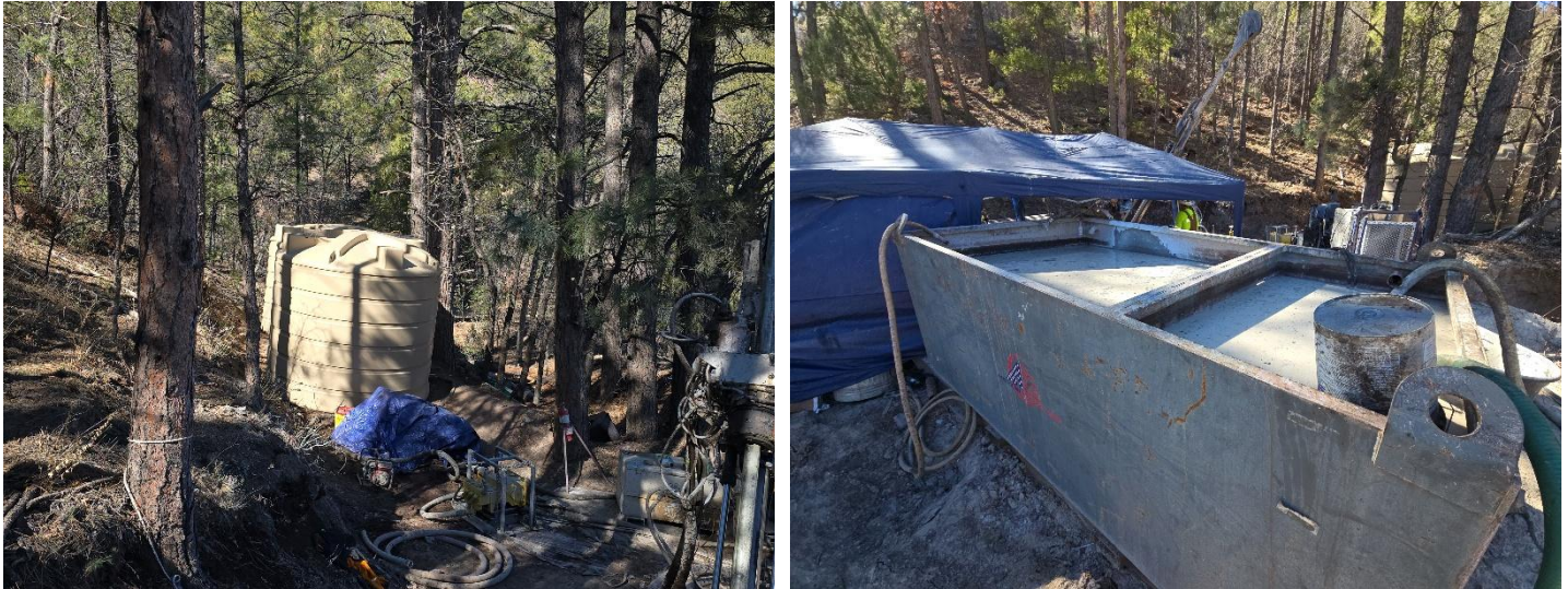
Figure 2 - Images from 2026 operations conducted under Summa's MMD Part 3 Permit at site DP04 depicting components of a closed-loop fluid management system showing mobile water tanks (left) and solids-control equipment (right).
