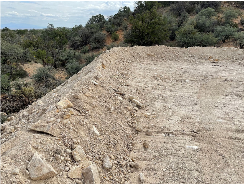
Image 8. Standard berms that will remain in place to prevent runoff from pads.
