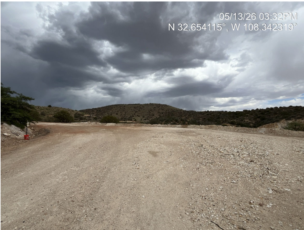
Image 2. Pad N status after drilling was completed and the sump was backfilled.
