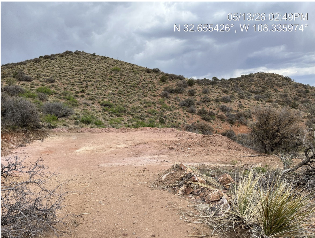
Image 6. Pad S status after drilling was completed and the sump was backfilled.
