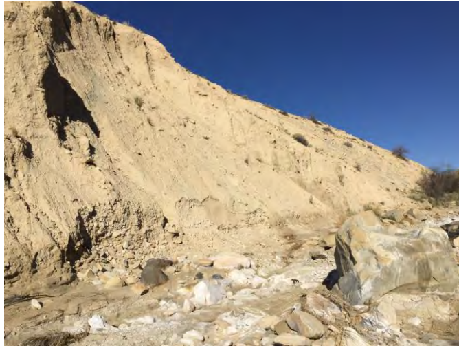
Figure 7: Large Failure Pile 3 at Approximate Station 68+00
