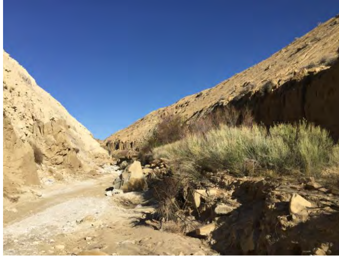
Figure 6: Large Failures of Pile 3 (Near Left) and Pile 4 (Far Center) at Approximate Station 65+00
