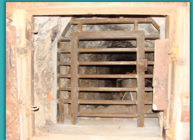
Before/After adit closure with bat gate: Cleveland Mine Safeguarding – Photos Courtesy of AML
