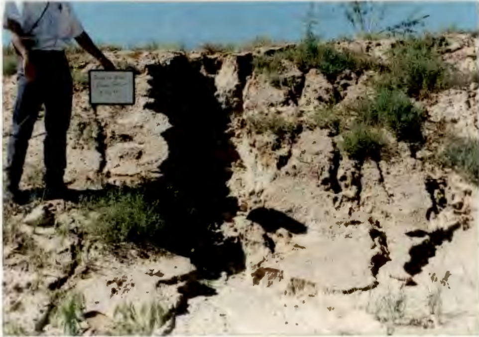
Isabella Mine, Erosion Feature, 9/12/95
