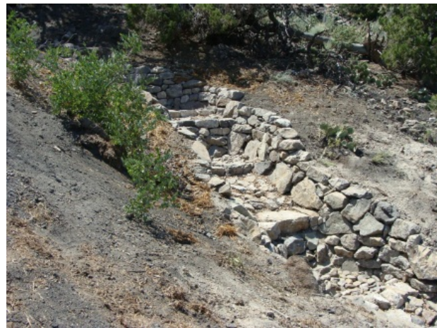
Figure 4: Recently completed, this Zuni bowl drop-structure was constructed for erosion control around the edge of a gob pile in Madrid.
