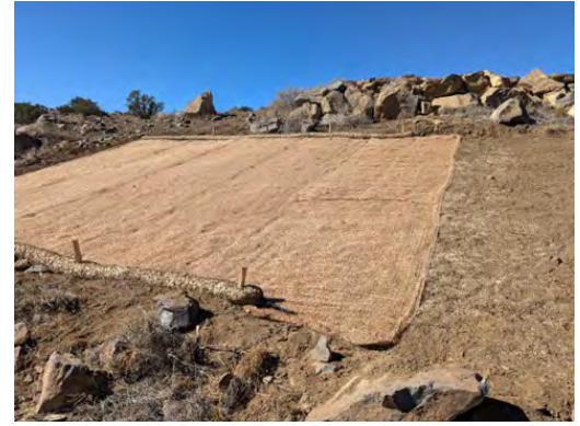
PHOTOGRAPH DEPICTING TYPICAL WATTLE AND BIODEGRADABLE MATTING.
