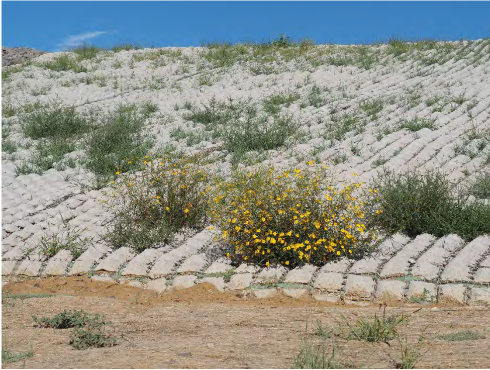
Photograph 86. Northwestern view, upslope, of the regraded, armored slope located at the transition from the reclaimed former borrow area to the reclaimed VS-10 (September 2025). Vegetation present on the concrete ECB. Some scouring noted at the slope toe.
