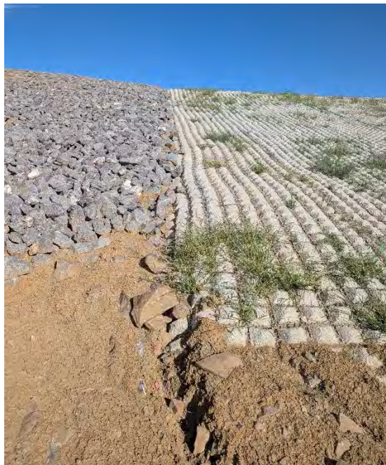
Photograph 87. View of the scouring present at the slope toe and concrete ECB anchor trench.
