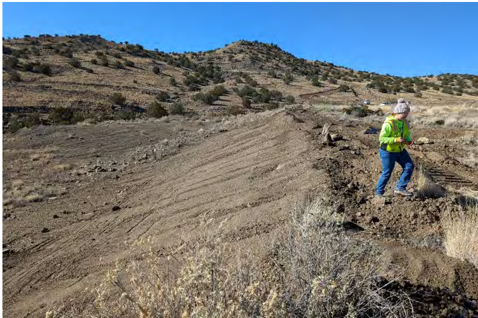
Photograph 15. The slope transition from the reclaimed Borrow Area to the reclaimed VS-10 had significant erosion, especially at the center, with a 3H:1V grade. Material was borrowed from the western slope portion (background) towards the foreground to the eastern portion of the slope to maintain an even 5H:1V grade (11-05-2024).
