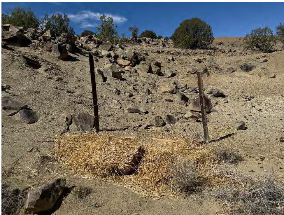
Photograph 81. Strawbales placed within channels along the drainage on the eastern side of the Reclaimed VS-12 area have started to degrade (April 2025).
