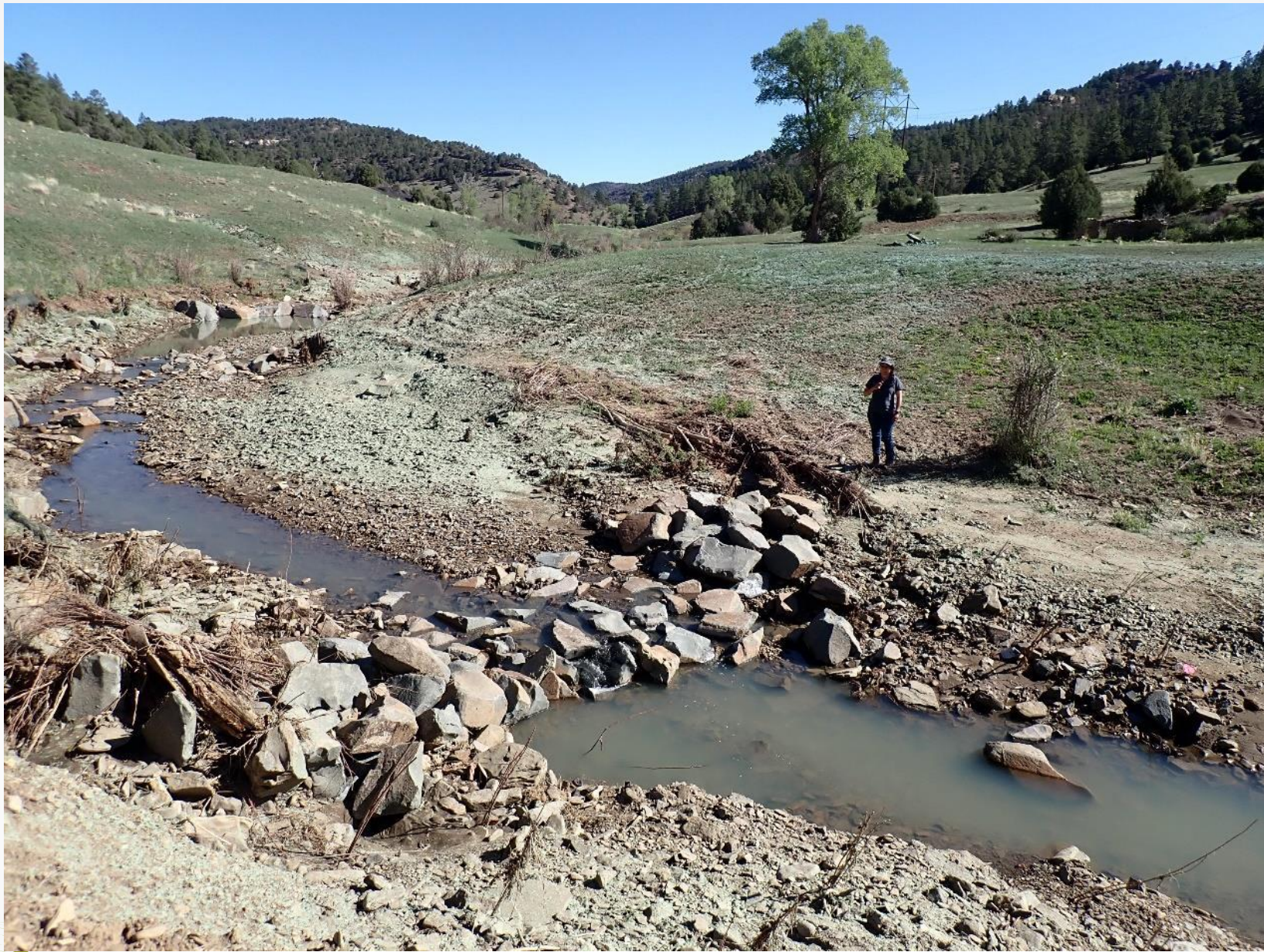
Figure 11. Structures doing their job after rain events, moving the flow away from eroding banks
