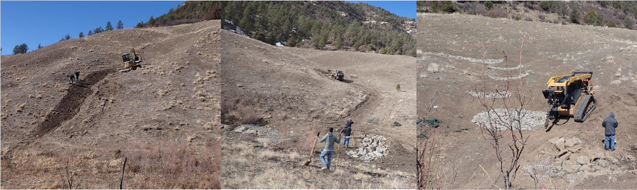
Figure 9. Shaping and installation of upland rock structures (one-rock check dams and media lunas)
