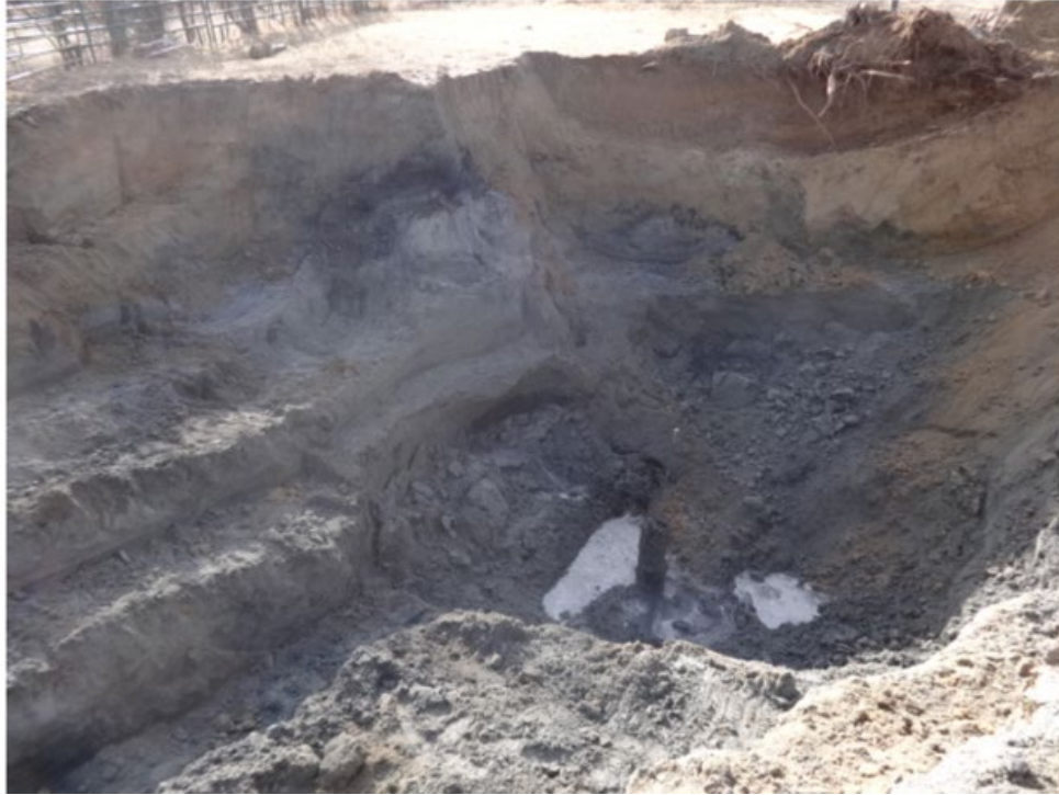
An orphaned well before plugging.
