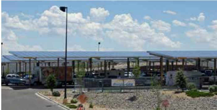
1 MW Solar Power Parking Lot at the Walmart Parking Lot in Truth or Consequences (Photo Credit: M. Gaiser)
