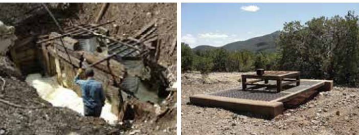
San Pedro - Polyurethane foam closure under construction San Pedro - Completed bat cupola
