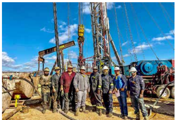
Thirty days after OCD received funds from the federal Infrastructure Investment and Jobs Act, crews began plugging an abandoned well just outside of Hobbs in Lea County. This funding will pay for plugging and remediation at 200 well sites across New Mexico over a twelve-month period.
