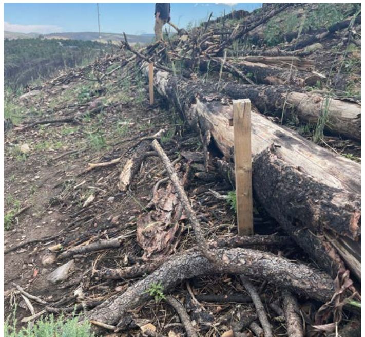
Well secured log erosion barrier. Image Credit: EMNRD
