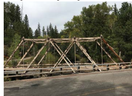
Image 2-53: Historic Pecos River Bridge (ca. 1921 CE, LA 50325) near NM Highway 63/Holy Ghost Creek Road; last remaining Howe Through Truss bridge design in NM
