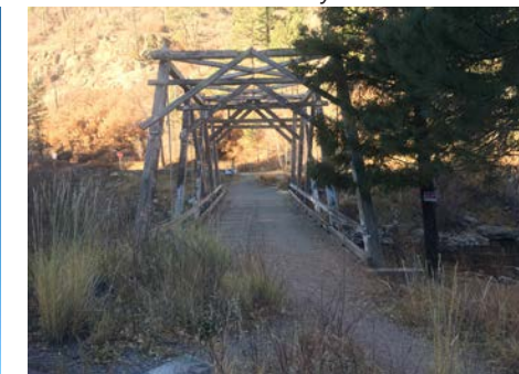
Image 2-17: Historic bridge at the confluence of the Pecos River and Holy Ghost Creek
