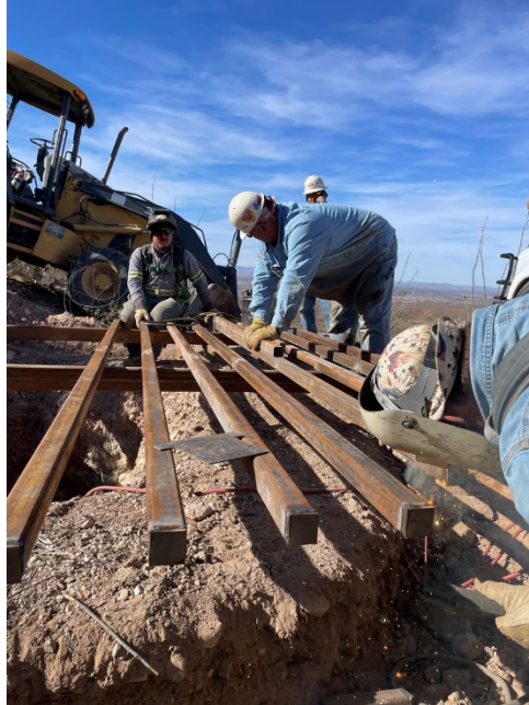
Safeguarding of a vertical shaft located immediately adjacent to a public access road.
