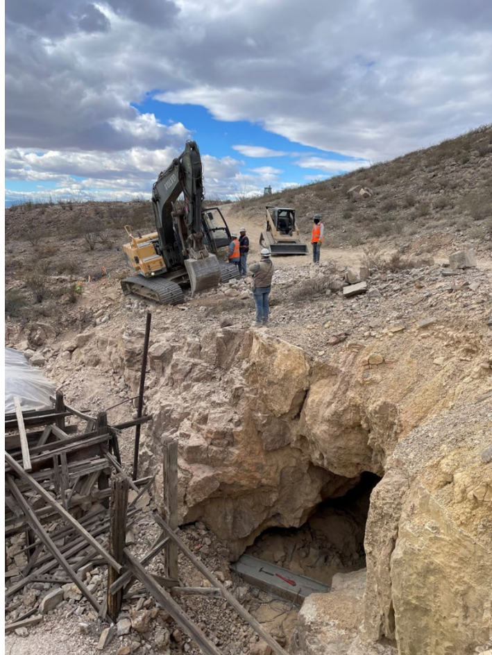
Crews working to backfill a dangerous mine opening while protecting the historical structure in place.
