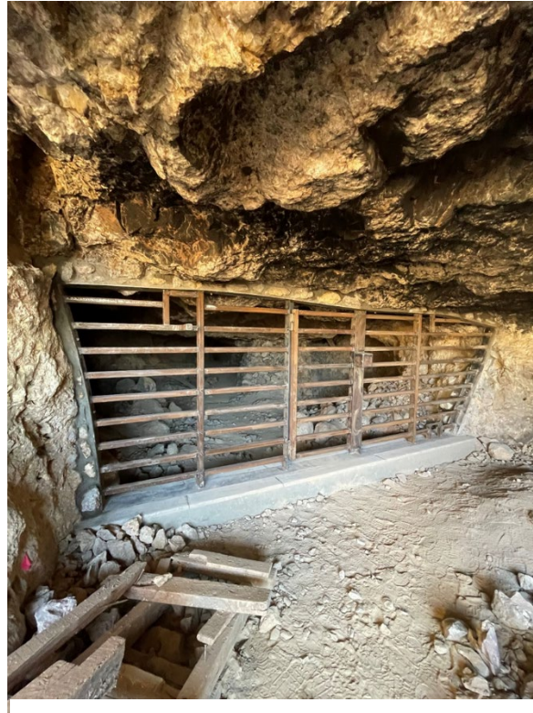
Bat-compatible safeguarding structure protecting the public from entrance into a horizontal mine adit.
