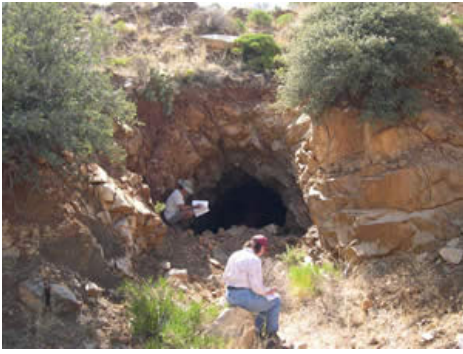
Abandoned adit with collapsing rock at the entrance.
