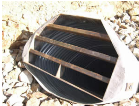
A culvert with a bat gate was constructed because bats were seen using the feature. The culvert is held in place with polyurethane foam.
