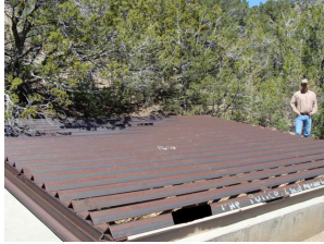
Water Canyon AML 4 Horizontal Bat Gate with Graffiti
