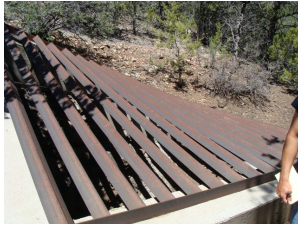
Water Canyon AML 2A Horizontal Bat Gate
