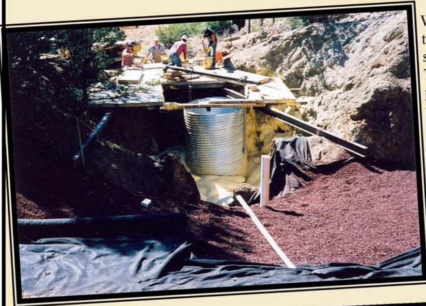
Polyurethane foam placement for the plug at the Tunia shaft; the scoria fill in the foreground has been placed over the polyurethane foam plug at the Tunia stope opening (See the cover photo for the completed installation)
